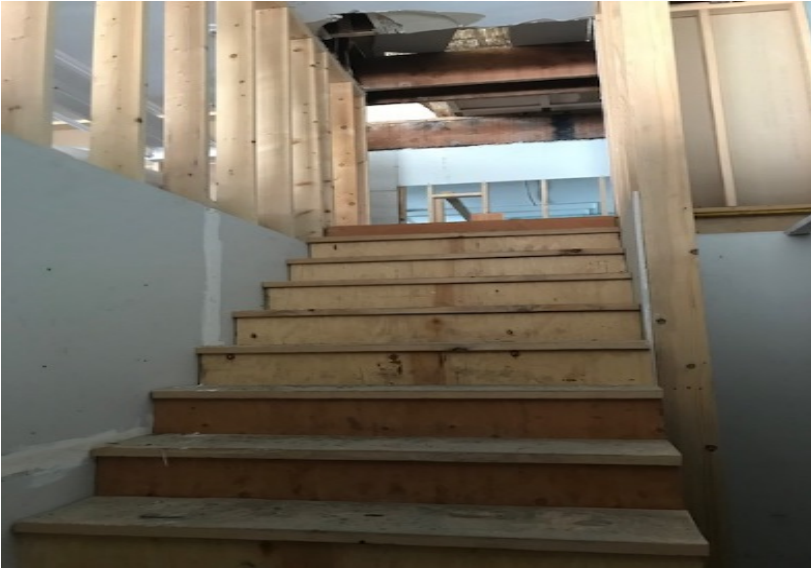
Ascending stairs built by former owner. The current owner indicated that the stairs were not completed/built to code.
