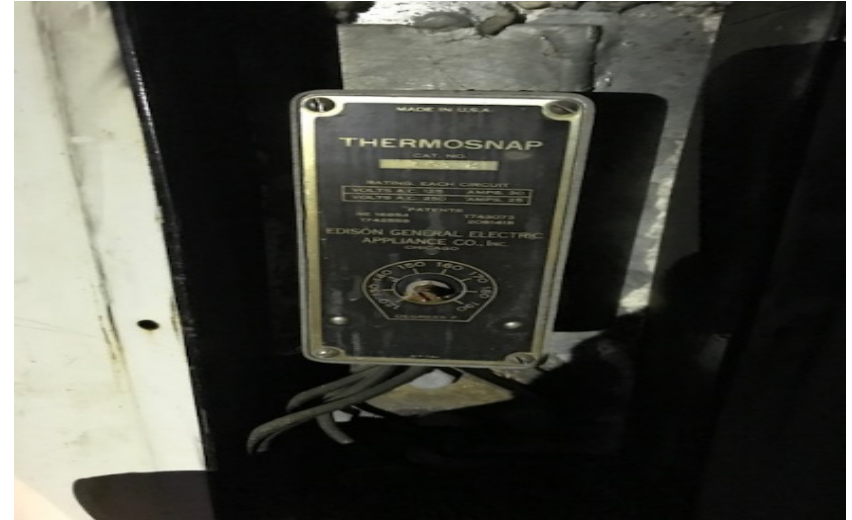
Hot water heater in basement. Water and power were not on during the time of the Site Reconnaissance and lighting was not ideal for quality photos. Potential asbestos wrap pipes were noted in the basement.
