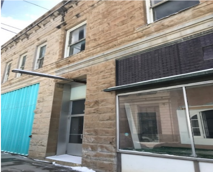
NE facing side of subject property and side entrance. The different colored stone denotes the non-subject property portion of the structure.
