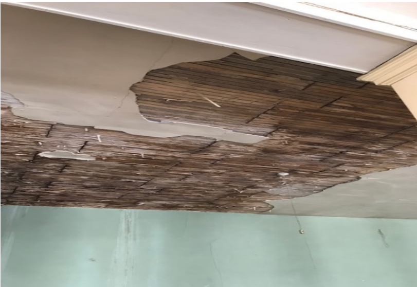
Area where plaster has been removed from the upstairs ceiling.
