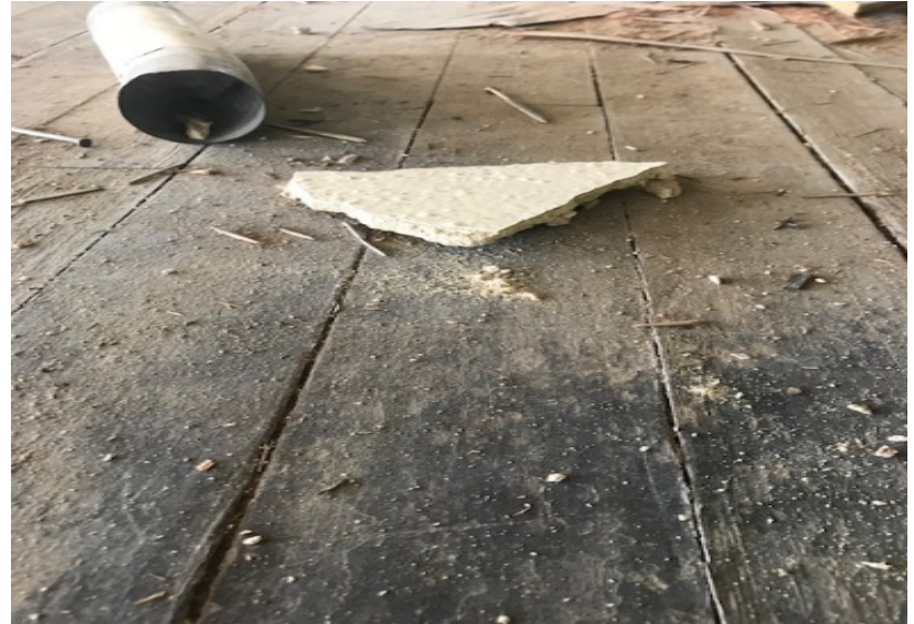
A segment of plaster that was removed from the upstairs ceiling.
