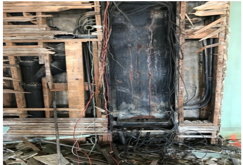
Electrical wire box and evidence of demolition activities.
