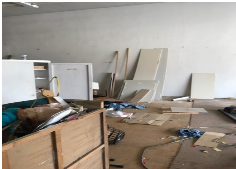
Inside of room intended to be/ or used as a "Sports Bar". Household debris and construction materials were observed.
