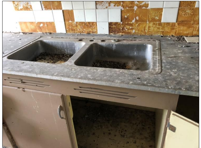
Stainless Steel Sink w/Insulation
