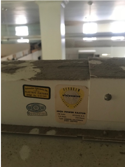
Fixture labeling on main floor.
