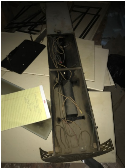
Lighting fixture in basement with presumed leaky PCB ballast.
