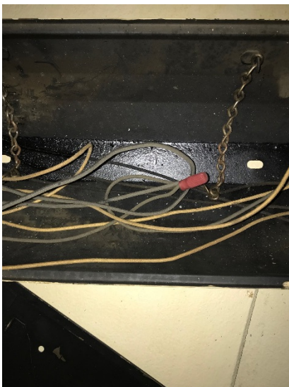
Lighting fixture in basement with presumed leaky PCB ballast. Note sheen indicative of a leak.
