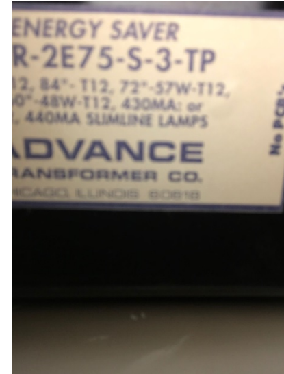
No PCB's labeling observed on a couple ballasts on main level.
