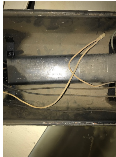
Lighting fixture in basement with presumed leaky PCB ballast. Note engraved ballast label.
