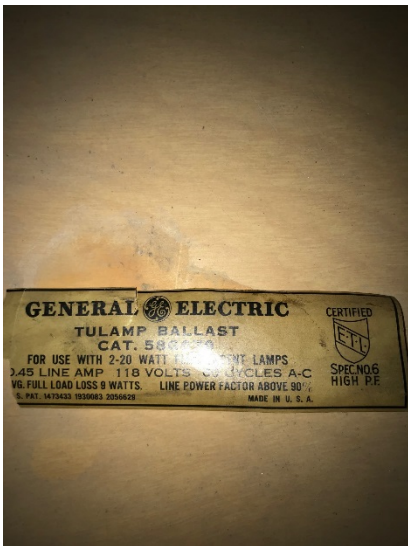
Lighting fixture in basement with presumed PCB ballast.
