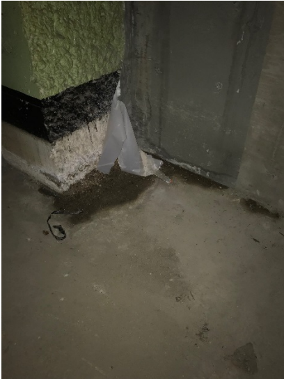
Evidence of water intrusion in basement: no mold observed.
