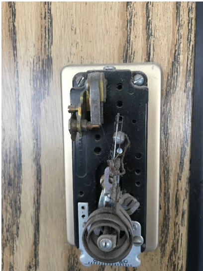
Thermostat on main level with mercury element not observed.
