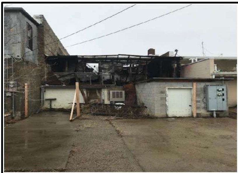
Figure 2: Photo from rear of building in alleyway showing burn damage.
